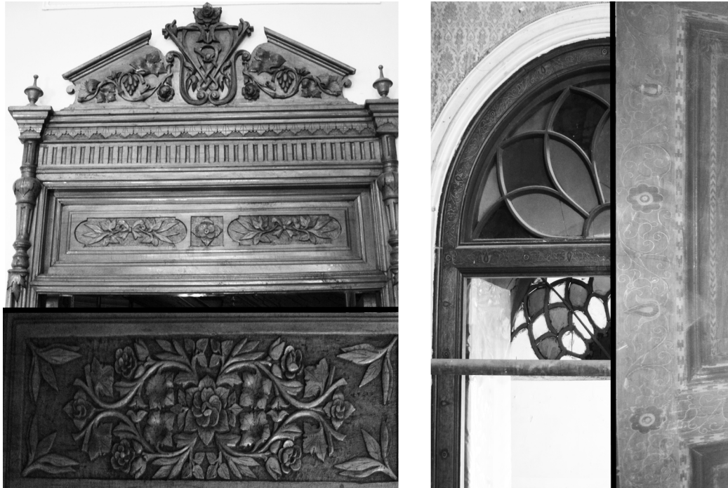
Fig. 15. The Door's Ornaments and Decorations of Mas'udieh's Divankhane and Grand Floor of Qavam Building
